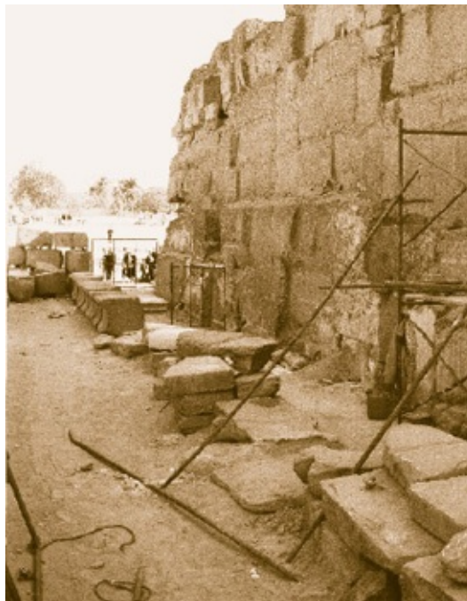
Figure 6.32. The eastern end of the north wall of the Valley Temple during restoration. We see piles of modern blocks of stone lined up to be placed and cemented against the base of the temple wall, which will forever obscure its true features and render impossible any closer reconstruction of what was going on here in the Old Kingdom. The Sphinx Temple is to the left of this photo and cannot be seen here. ( Photo by Robert Temple )
