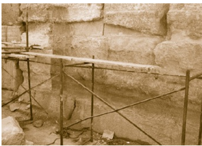
Figure 6.31. The north wall of the Valley Temple undergoing restoration. Modern pieces of limestone have been cut and inserted into holes; cement has been smeared all along depressions to even them out. All traces of anomalies are being erased. This is despite the fact that tourists never come here and never will. The horizontal lines showing ancient water erosion run along the lower wall at a level above the base blocks. ( Photo by Robert Temple )
