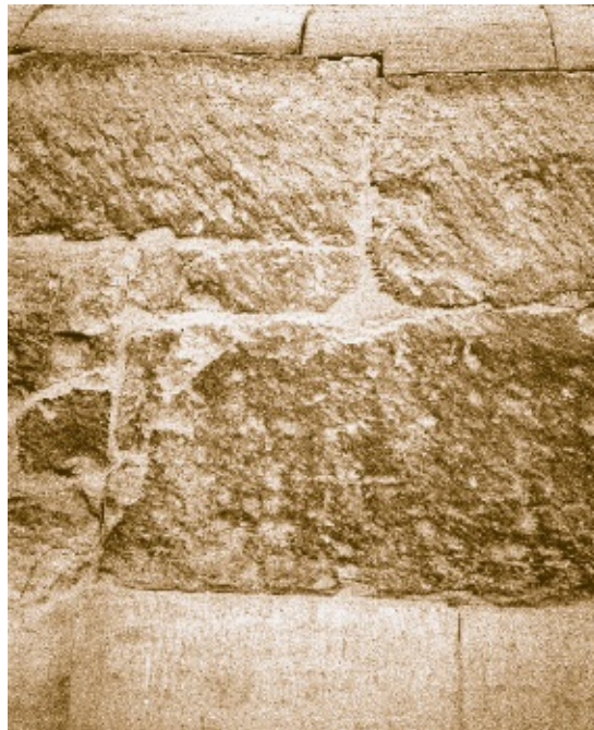
Figure 1.35. A close-up of some of the restoration on the Sphinx. The central limestone blocks are believed to be of Old Kingdom date, from the first repair job, but modern cement has been smeared into the cracks between them. Above them have been laid modern limestone pieces, carefully fitted to the surface, and below, larger limestone blocks have been cut and inserted into holes where older blocks had fallen out and been lost. (Photo by Robert Temple)
