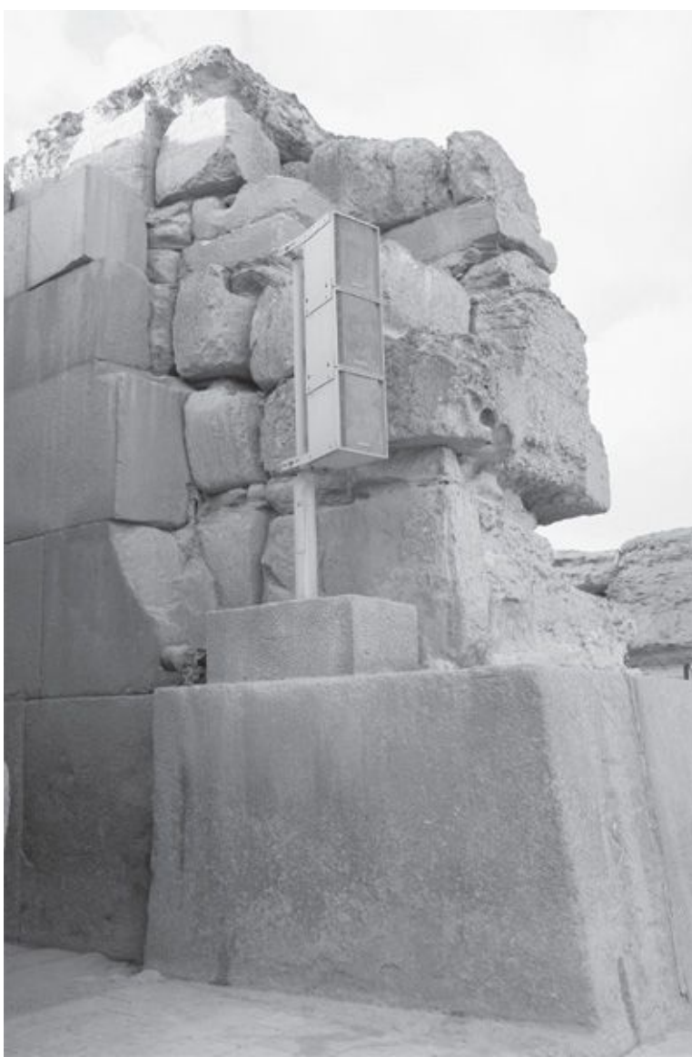
Fig. 7.12. Smooth granite ashlars (Fourth Dynasty?) facing the older weathered and eroded limestone core blocks of the Valley Temple. (Photo courtesy of R. Schoch and C. Ulissey.)
