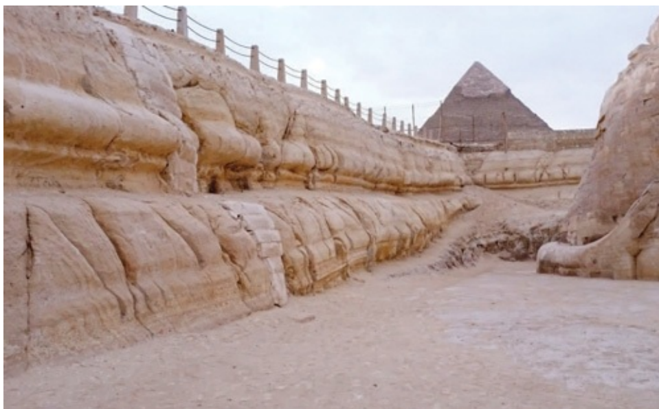
Plate 12. The southern wall and southwestern corner of the Sphinx Enclosure showing the extreme water weathering and erosion from rain and water runoff (an undulating profile with deep vertical fissures). Note the modern repair to one of the fissures. (Photo: R. Schoch & C. Ulissey.)
