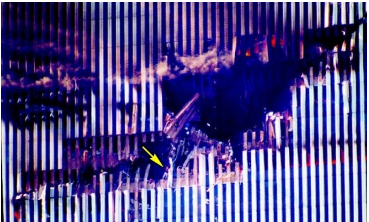
Detailed view of the damage supposedly inflicted by the alleged passenger “Boeing-767” to the WTC North Tower’s steel perimeter columns (a live person could be seen there, in addition).
