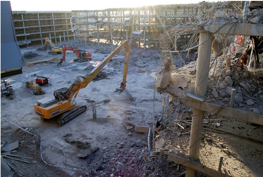
Above – destroyed car-parking at the Terminal 4 Madrid Barajas airport at the end of clean-up operation.
