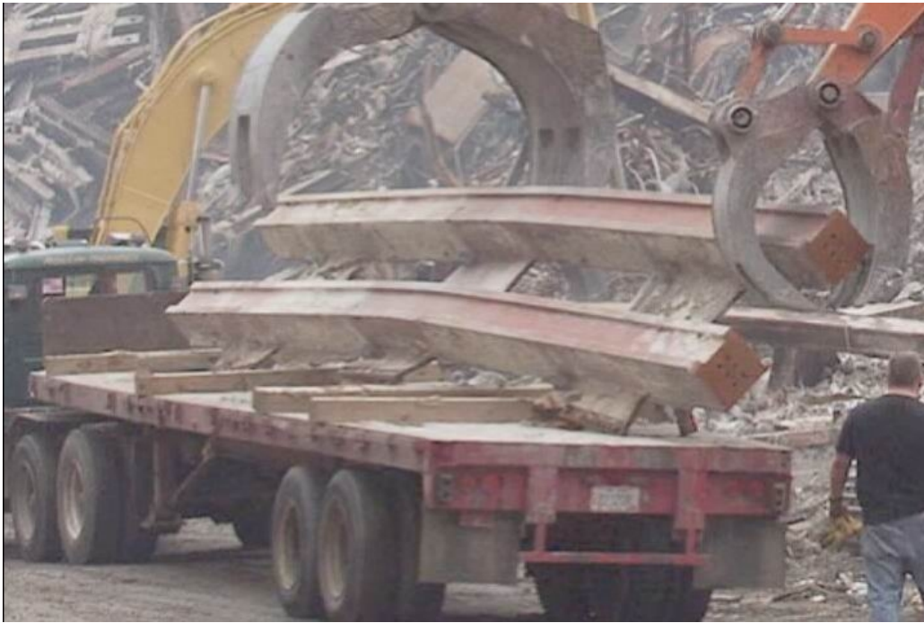
Above – perimeter columns of the Twin Towers being loaded onto a truck at “ground zero”.
