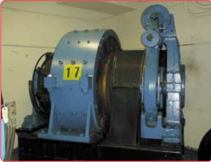
Shuttle elevator hoist machine
