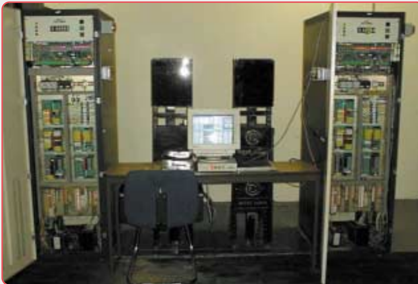
Elevator machine room showing typical installation of SWIFT controller
