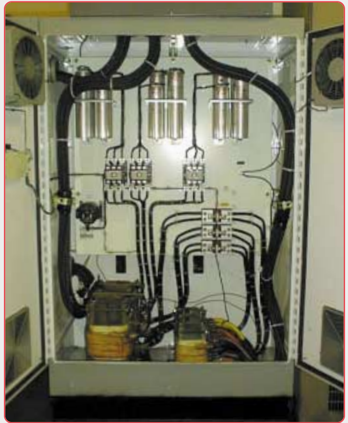
The harmonic filter installed in motor generator room
