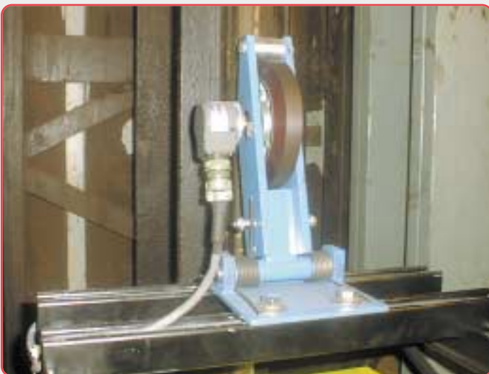
Top of shuttle elevator car showing rail-mounted encoder
