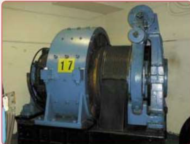
Shuttle elevator hoist machine
