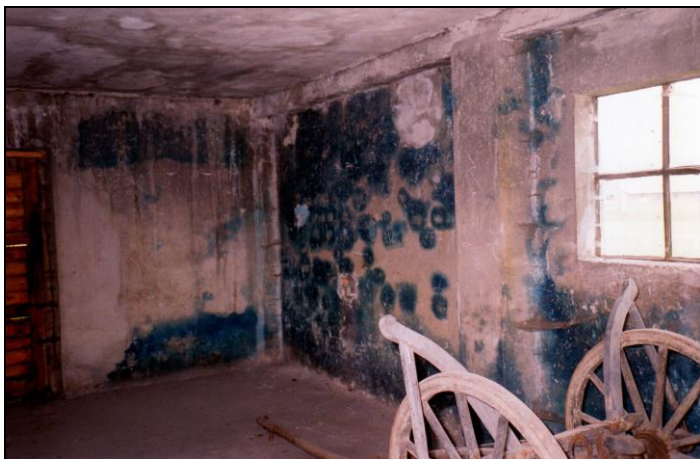
Illustration 20: Blotchy blue discoloration of the inner walls – from the floor to the ceiling – of the Zyklon B disinfestation wing of Hygiene Building 5a in Birkenau, Construction Section I (© Carlo Mattogno 1992).
