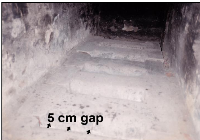
Illustration 37: Interior of the Topf Company furnace, type Auschwitz, with slits in the fireclay grate with a width of merely 1.97 inch.
