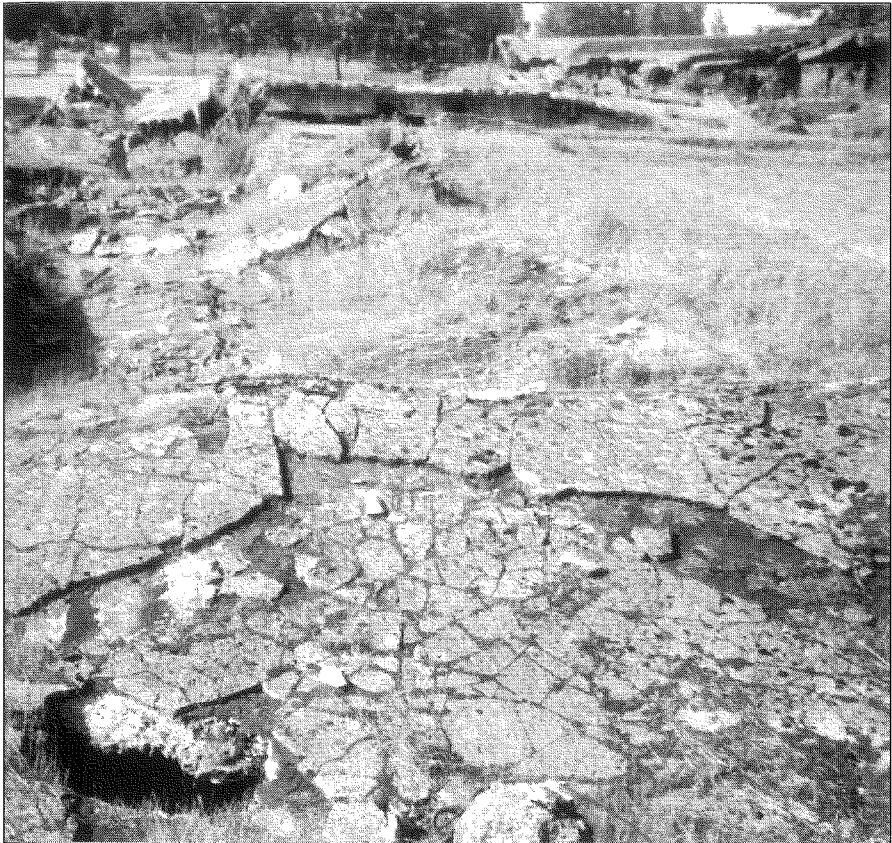
Illustration 15: The collapsed reinforced concrete roof of morgue #1 of Kremas 2 at Birkenau in August 2000.
