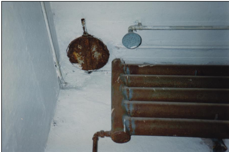
Photo 7: “Gas chamber” at Mauthausen: Lid of the ventilation opening and part of the radiator. December 1990. © Carlo Mattogno.
