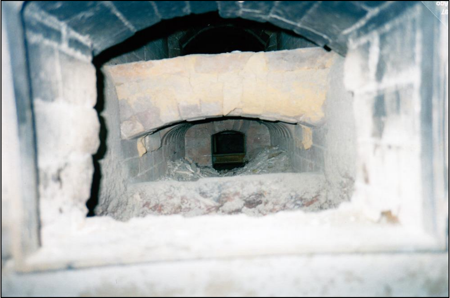
Photograph 313: Inside of a furnace seen from the gasifier's coke-loading door. Foreground: the gasifier; behind it: the ash chamber with the ash doors in the background; above that: the muffle's fireclay grate; top: the muffle.
