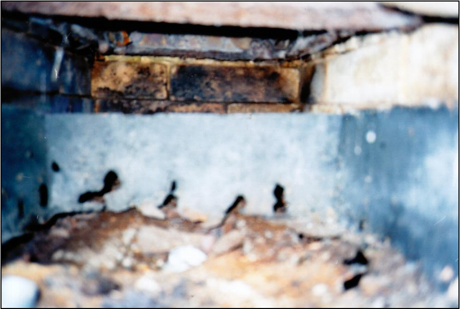
Photograph 355: as above; inside of the ash chamber seen through its rear service door, with the corroded iron ash container.
