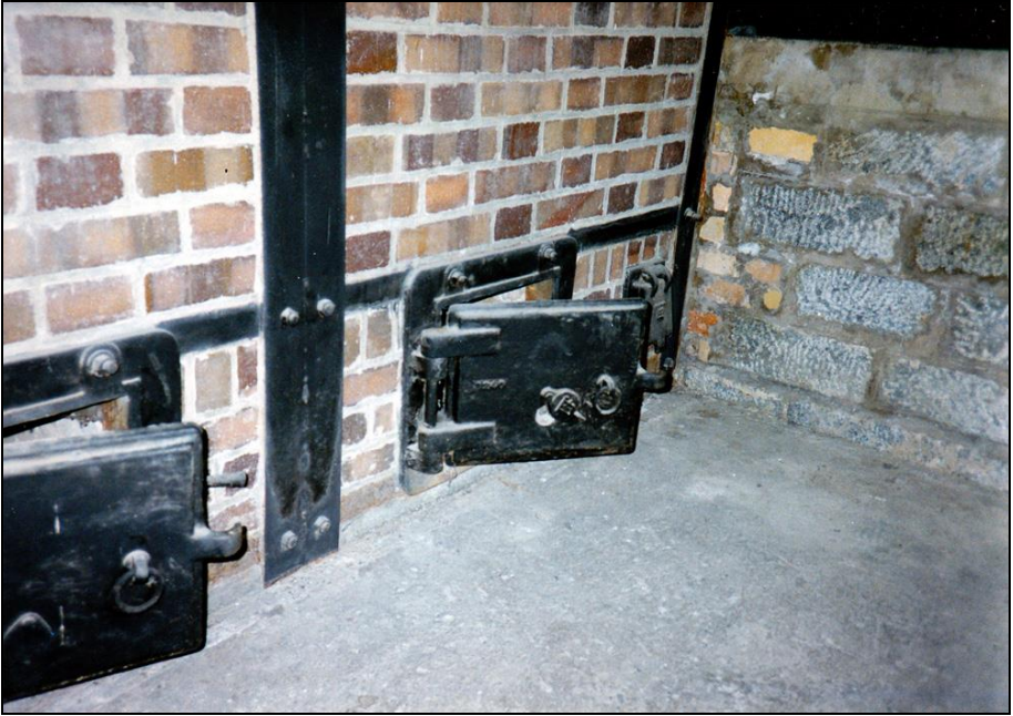
Photograph 80: as above, the gasifiers' ash-chamber doors.
