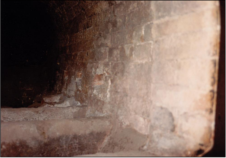
Photograph 147: as above, right-hand square openings of the combustion-air feed. Bottom: muffle grates.
