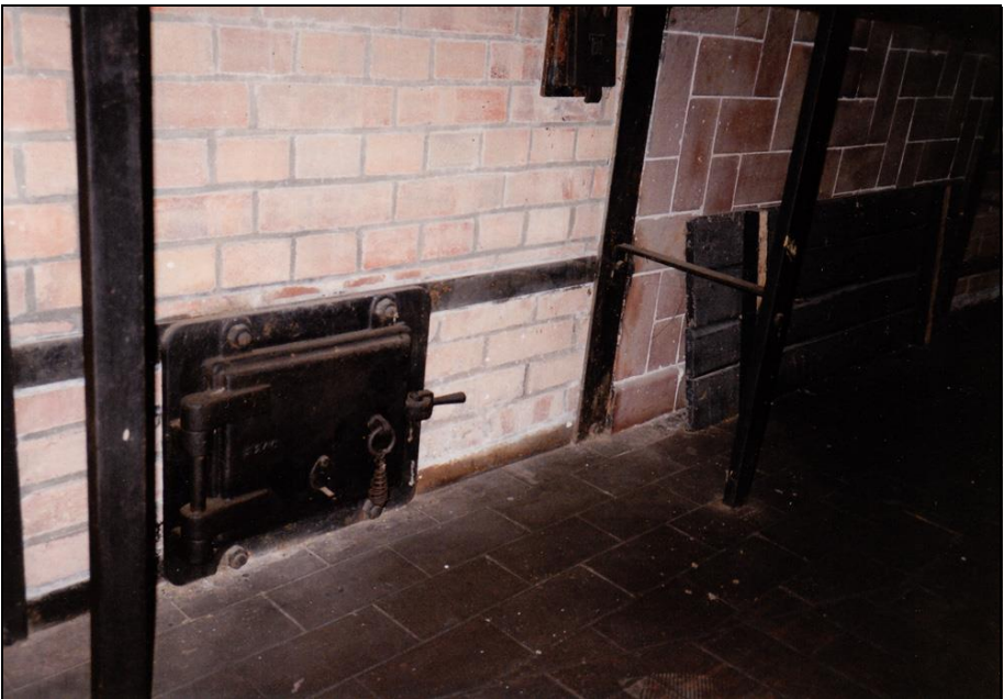
Photograph 176: as above, left-hand muffle: the gasifier's ash-chamber door (bottom) and its combustion-air-channel door (top right).
