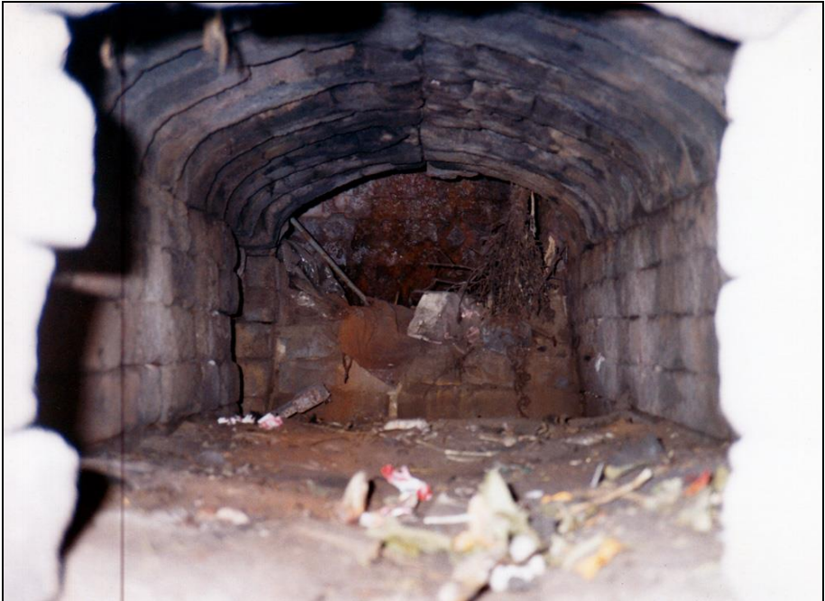
Photograph 273: The ash chamber of the left-hand muffle. Top: underside of the muffle's grate bars. On the left wall: opening connecting it with the auxiliary hearth. At the back: the gasifier's pit.
