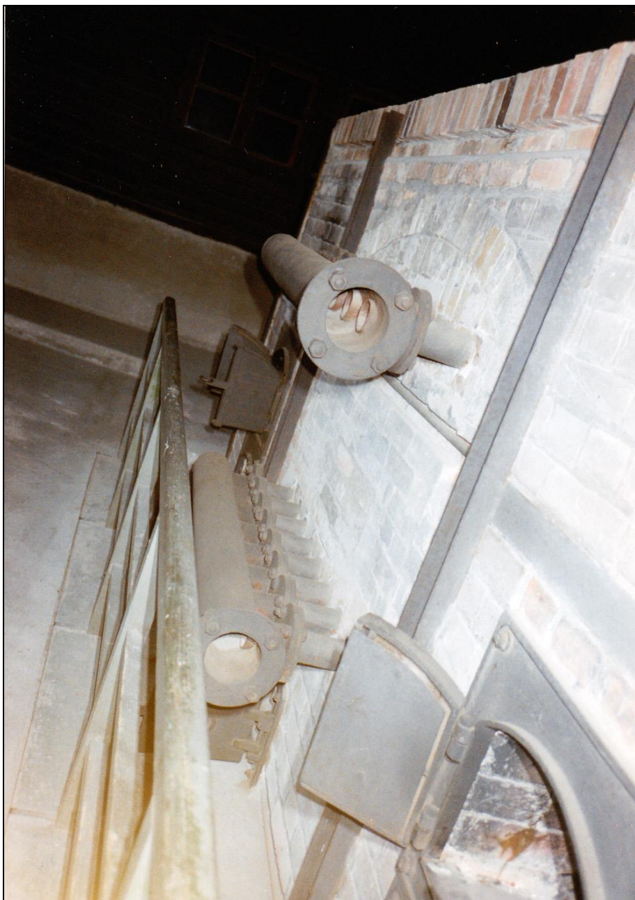
Photograph 308: as above. Hot-water pipes of the recuperator.
