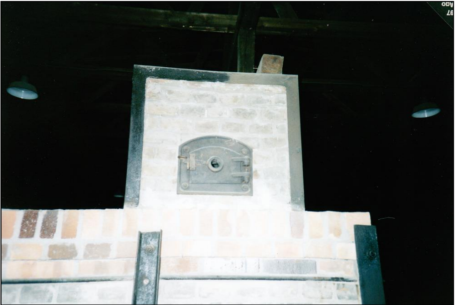
Photograph 310: as above, smoke duct with inspection door.
