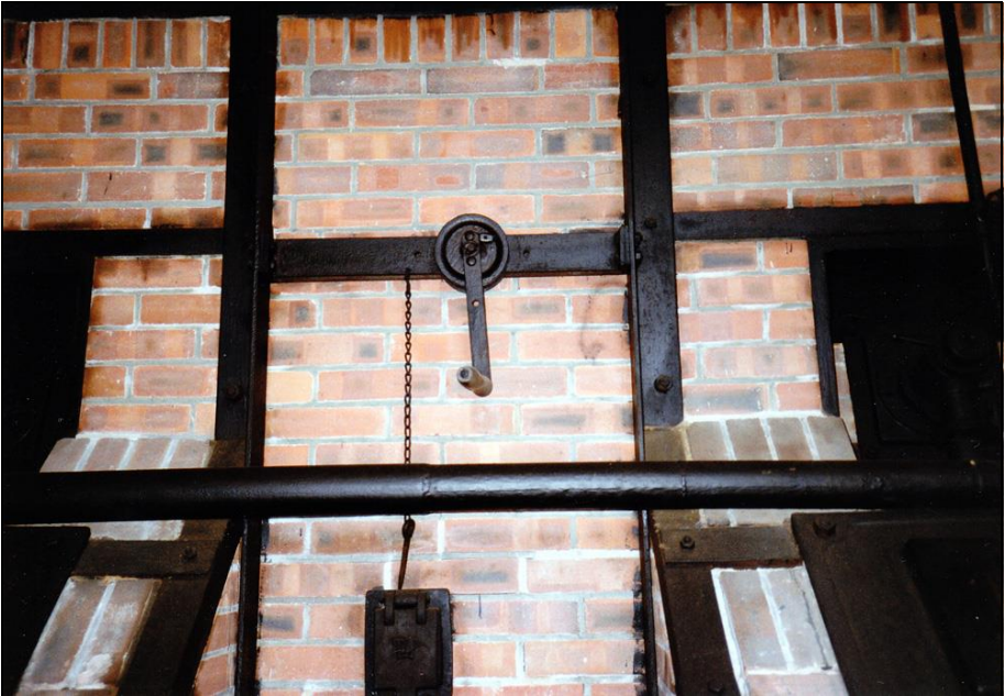
Photograph 168: as above, central muffle. Crank operating the smoke-duct damper (top) and the door to the muffle's rear combustion-air channel.
