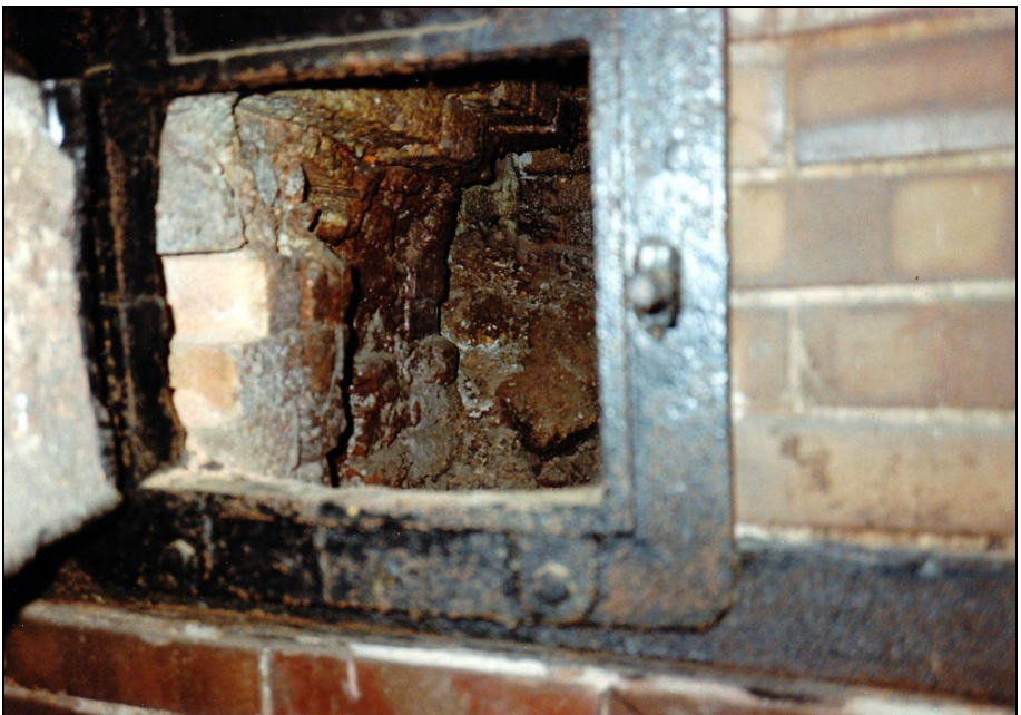
Photograph 9: Right-hand gasifier: coke-loading door.
