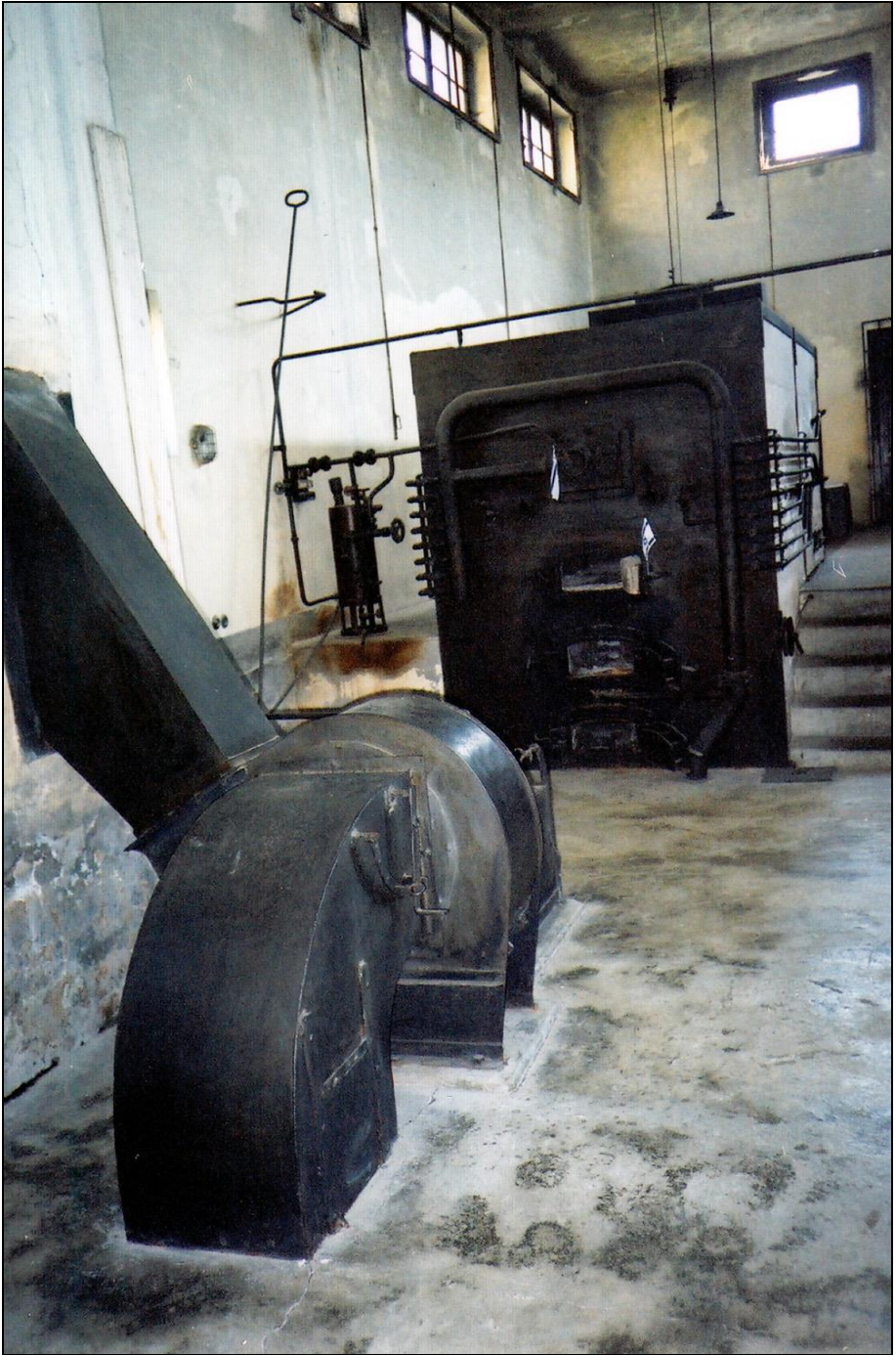
Photograph 357: as above, side view.
