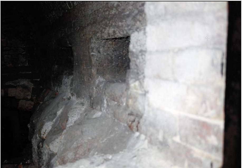
Photograph 134: as above, right-hand muffle wall with rectangular openings connecting this side muffle to the center muffle.
