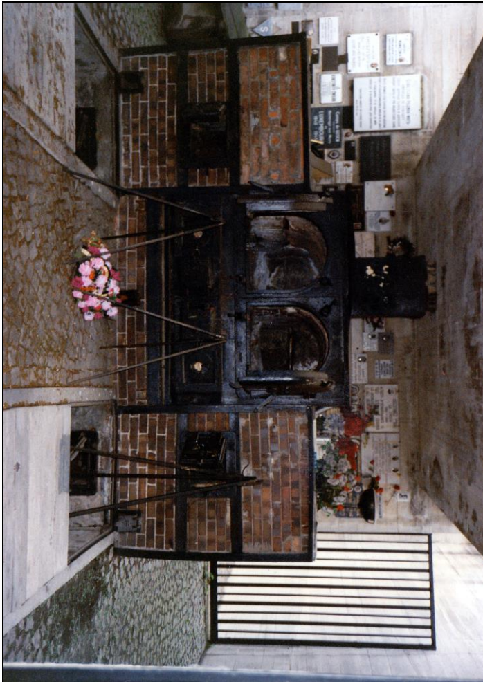
Photograph 1: Original furnace body made of coated sheet metal with added masonry gasifiers at both sides.
