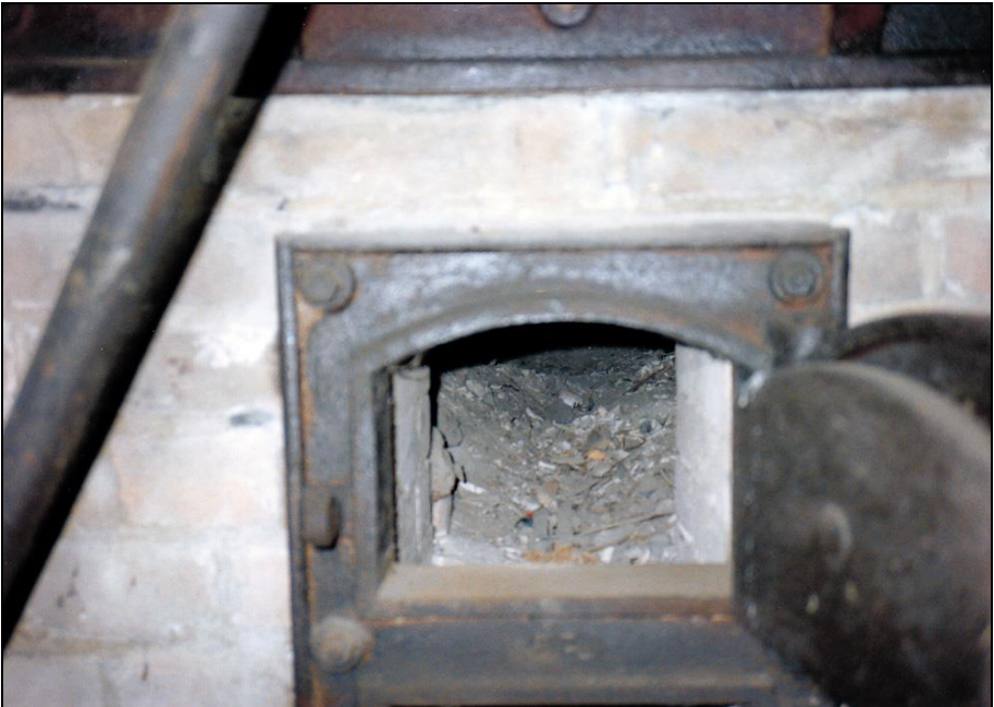
Photograph 303: Access door to the post-combustion area.
