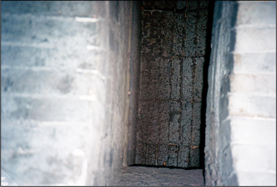
Photograph 302: Vertical duct of the flue-gas outlet.
