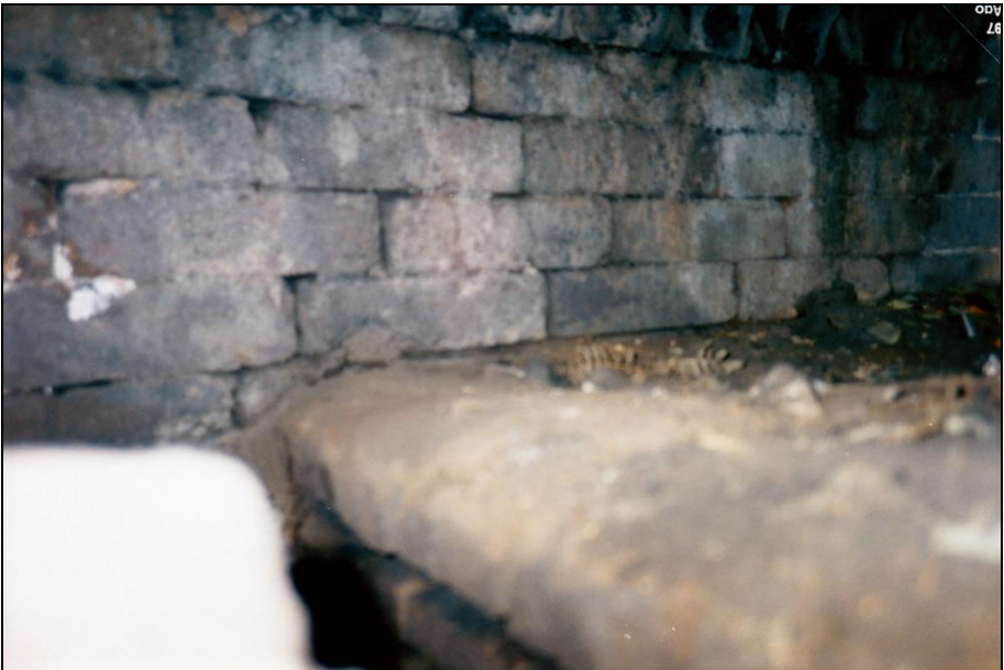
Photograph 282: as above. The muffle's ash chamber seen through the auxiliary gasifier's ash-chamber door.
