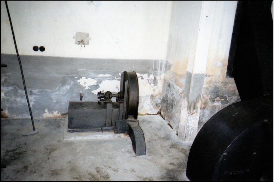
Photograph 358: Combustion-air blower for the left-hand furnace of the front pair.
