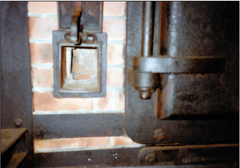
Photograph 152: as above, the ash chamber's combustion-air-supply channel.
