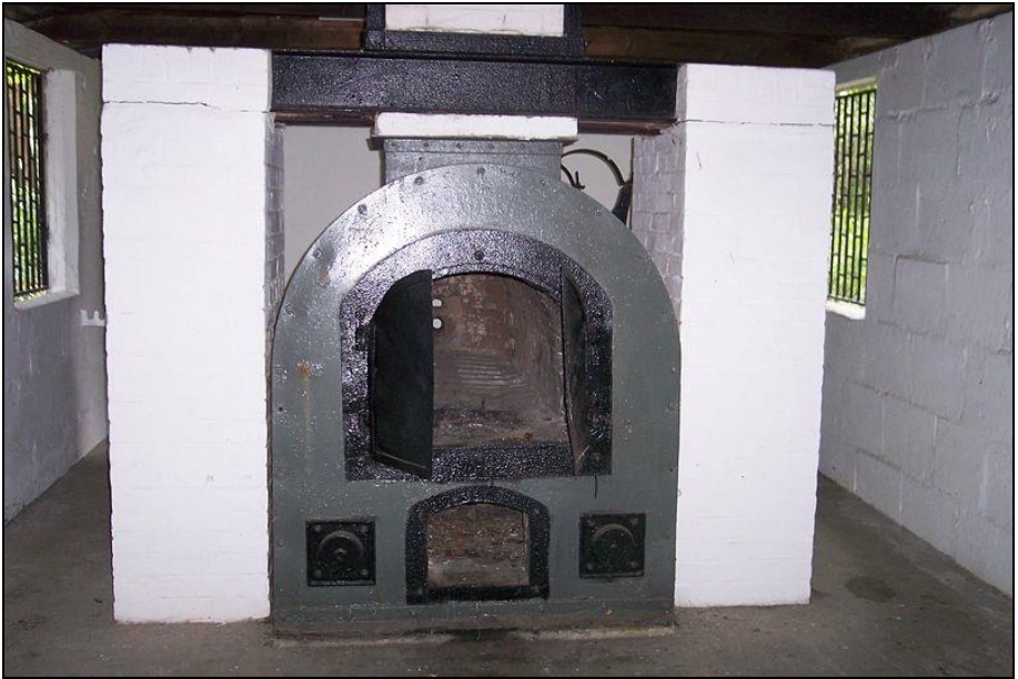
Photograph 331a: Naphtha-fired cremation furnace at Blechhammer sub-camp.
