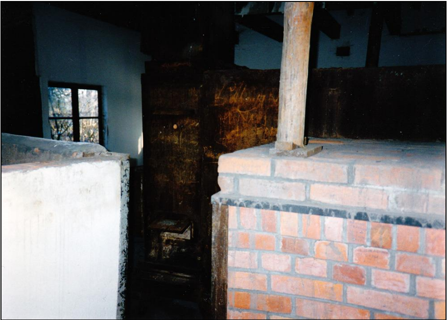
Photograph 50: Left-hand side of the furnace; background: open service door for the pilot flame at the chimney's base.
