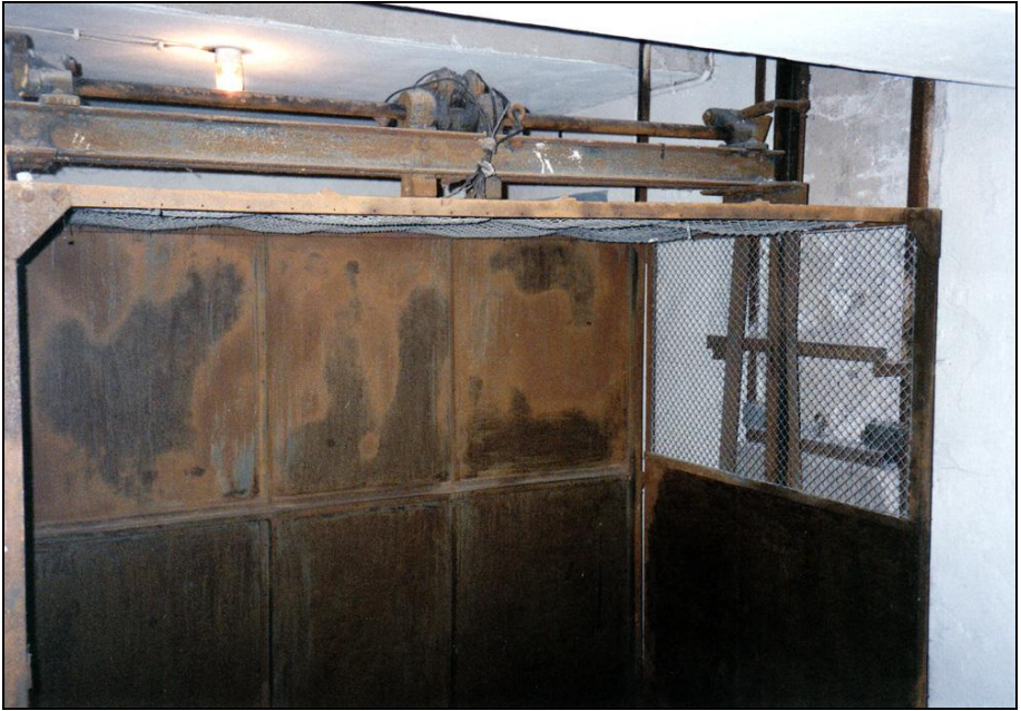
Photograph 212: as above, freight elevator, front.
