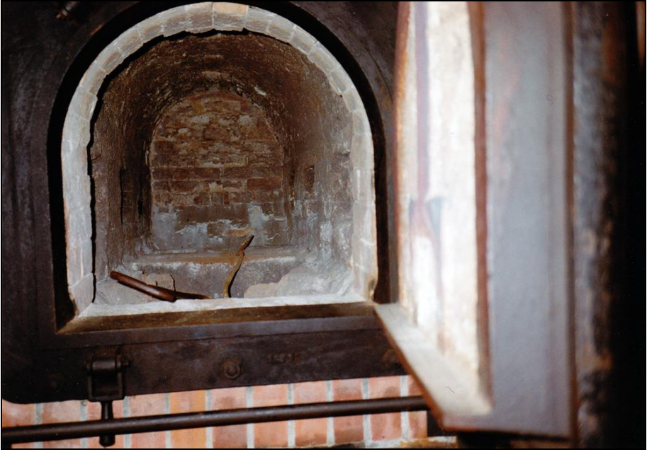
Photograph 135: as above, central muffle. Both side walls have three rectangular openings connecting it to the side muffles.
