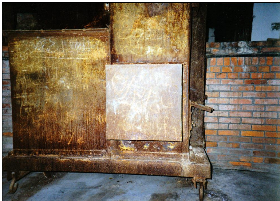
Photograph 47: Rear view of the furnace; base of the chimney with an open service door at the right-hand side. The square metal sheet welded to the chimney's bottom closes the opening for the original forced-draft blower.
