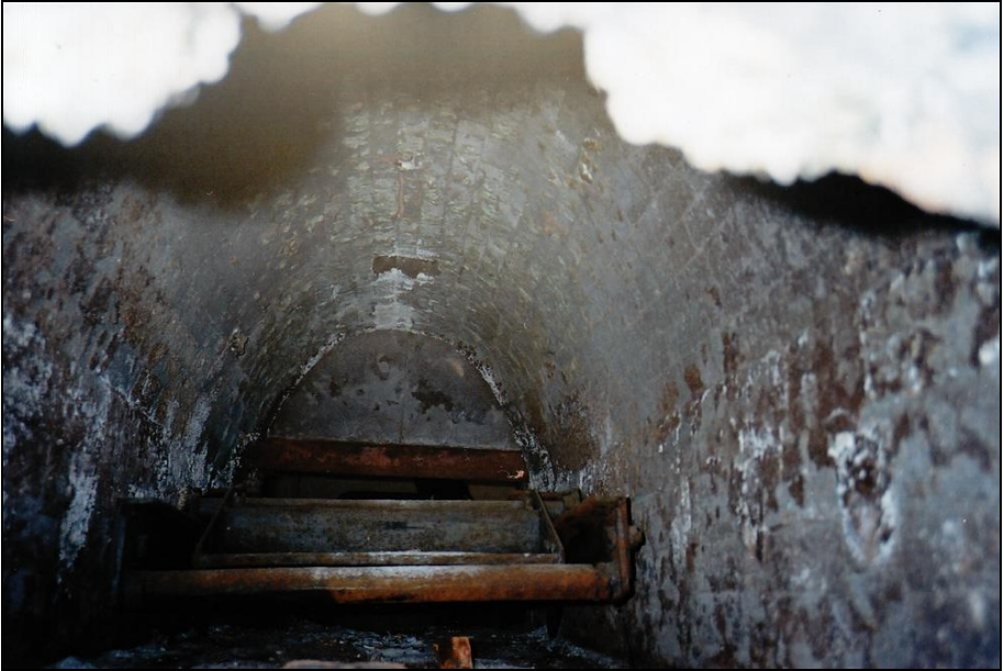
Photograph 352: as above; the muffle's inside seen from its rear service door. In the foreground the front part of the corpse-introduction cart.
