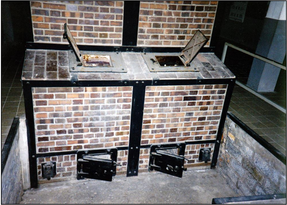
Photograph 78: Rear side of the furnace with the gasifiers sporting the coke-loading doors (top) the ash-chamber doors (large door at center bottom) and the combustion-air-intake doors (bottom, small doors).
