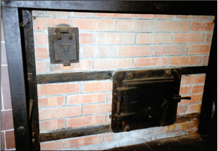
Photograph 173: as above, right-hand muffle. The gasifier's ash-chamber door (bottom) and the door of the gasifier's combustion-air channel (top left).
