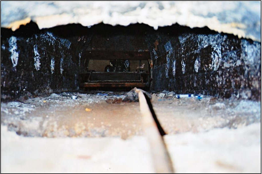
Photograph 353: as above, with the introduction cart pulled out. In the foreground, the shaft of the scraper to move cremation remains.
