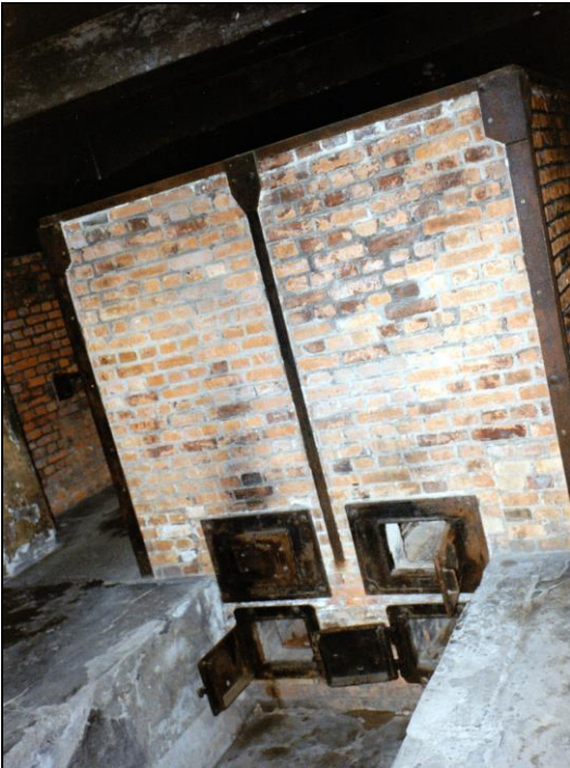
Photograph 97: Furnace no. 1, rear side. The furnaces were reconstructed without gasifiers. The gasifiers' coke-loading doors are therefore necessarily in the wrong position over those of the ash-chamber doors. See Photo 78.
