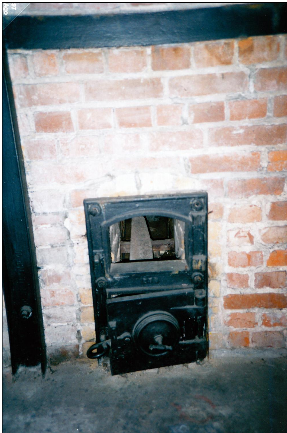
Photograph 280: Left-hand furnace; doors of the auxiliary gasifier.
