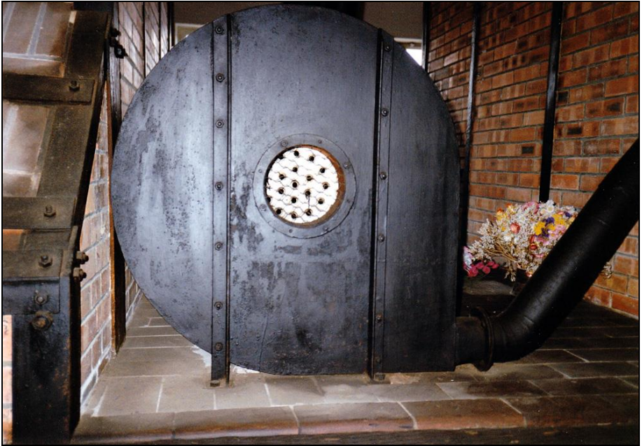
Photograph 195: Combustion-air blower for the oil burner of the furnace heated with either naphtha or coke. Rear view.
