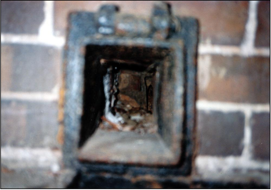
Photograph 6: Left-hand gasifier's primary air intake.
