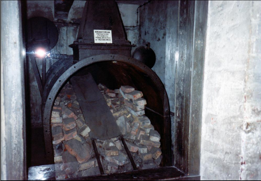
Photograph 330: Front view of the furnace. The interior of the furnace was completely destroyed. At the top the conical chimney (center), the blower (left) and the naphtha tank (right).
