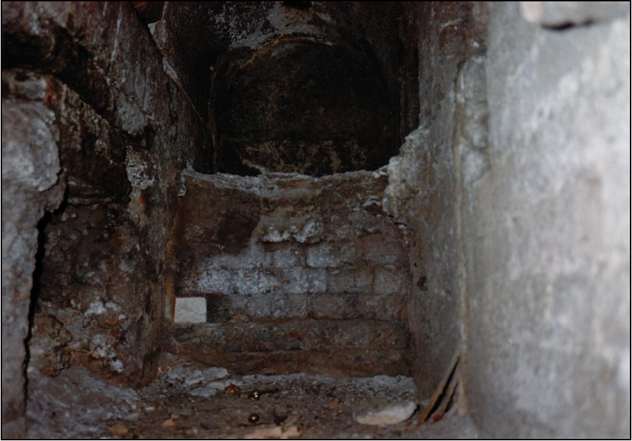
Photograph 18: Left-hand muffle: ash compartment. Visible at the bottom left is the first opening connecting it to the gasifier.
