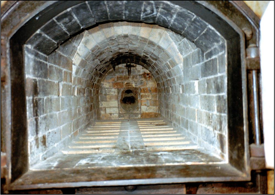
Photograph 320: Inside of the muffle. Bottom: the refractory grate; on the back wall: the main burner's nozzle; on the side walls: openings of the combustion-air-supply channels.
