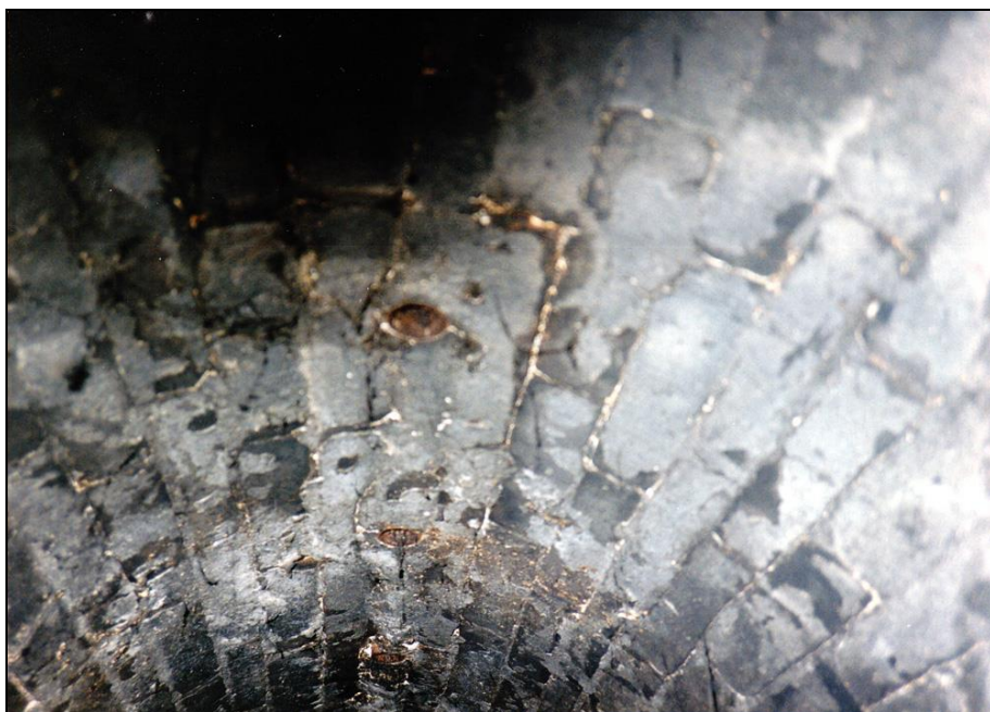
Photograph 61: Vaulted ceiling of the right-hand muffle; outlets of pipes connected to the blower.
