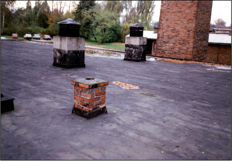
Photograph 104: Roof of Crematorium I: The two ventilation chimneys of the cremation furnaces (black and grey).
