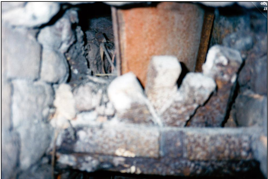
Photograph 277: Inside the right-hand furnace's main gasifier viewed through the ash-chamber door. The hearth's grate has been damaged, with only four remaining bars leaning against the outer support bar.
