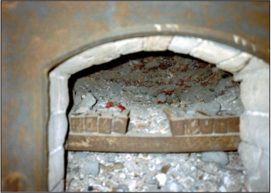
Photograph 311: The gasifier grate.
