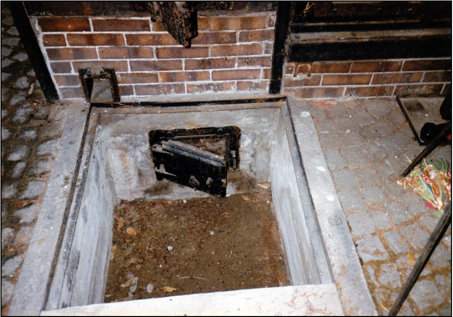
Photograph 7: Left-hand gasifier: slag/ash-removal door and service pit.
