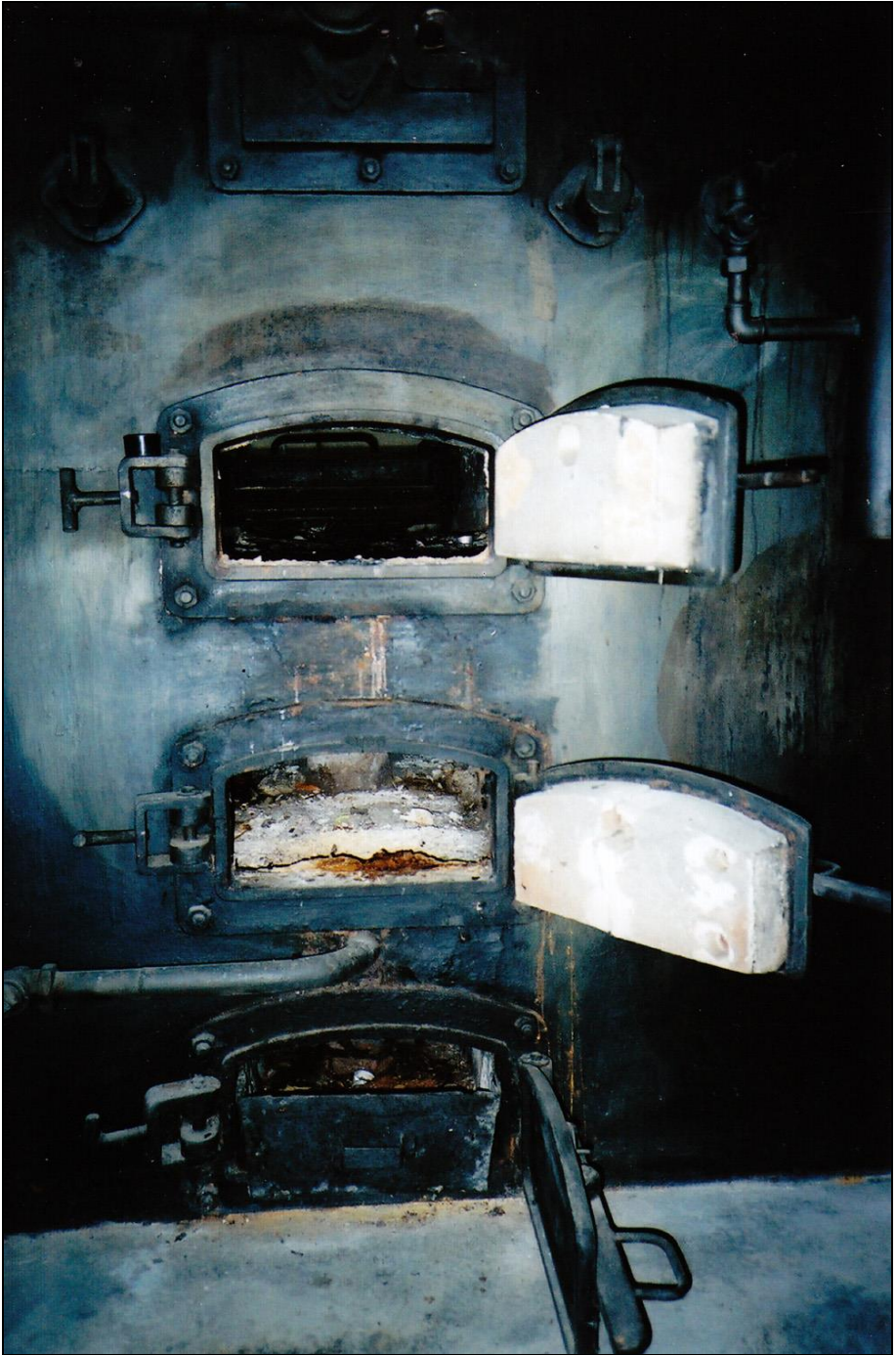
Photograph 351: Left-hand furnace of the front pair, rear view; the three service doors: for the muffle (top), the post-combustion chamber (center) and the ash chamber with the ash receptacle (bottom).
