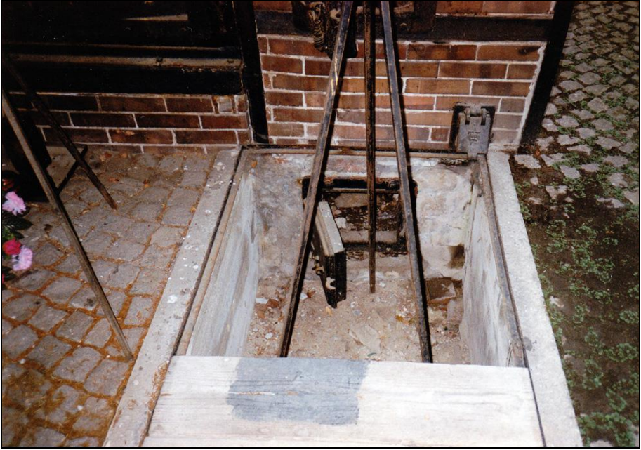
Photograph 10: Right-hand gasifier: primary air-intake door, ash-removal door and service pit.
