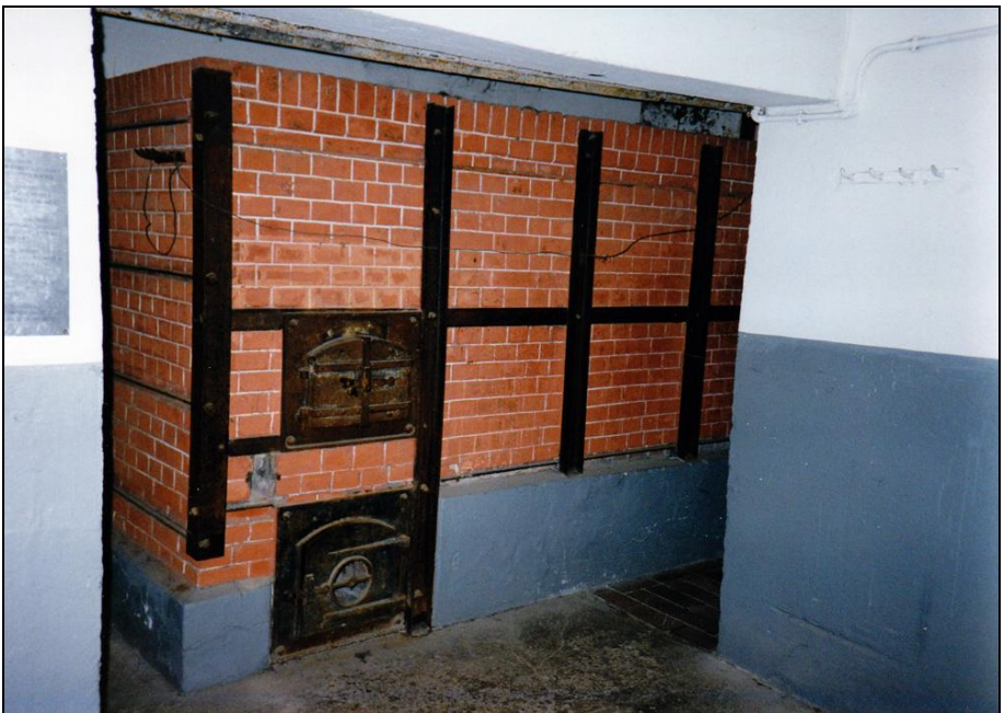
Photograph 245: left-hand side view; the gasifier's coke-loading door (top) and ash door (bottom).
