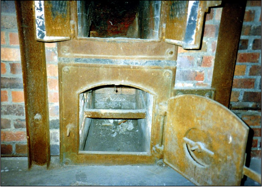
Photograph 262: Ash-chamber door of the main gasifier.
