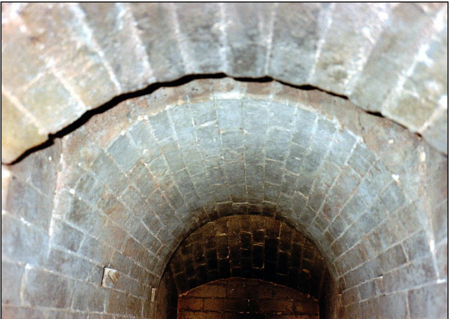
Photograph 321: as above; the vaulted muffle ceiling with the smoke-duct opening in the foreground.
