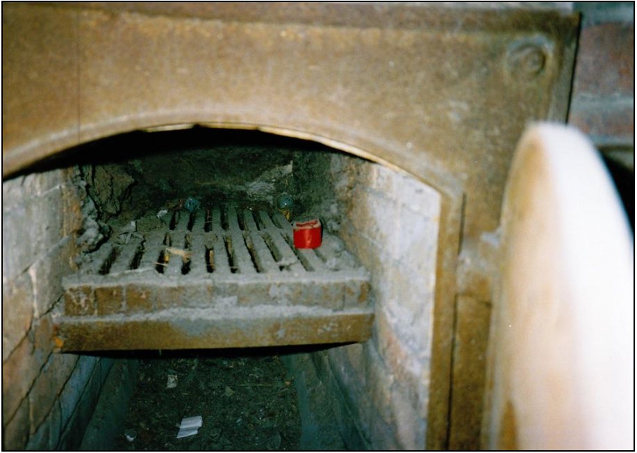
Photograph 264: View through the main gasifier's ash-chamber door onto the coke grate.
