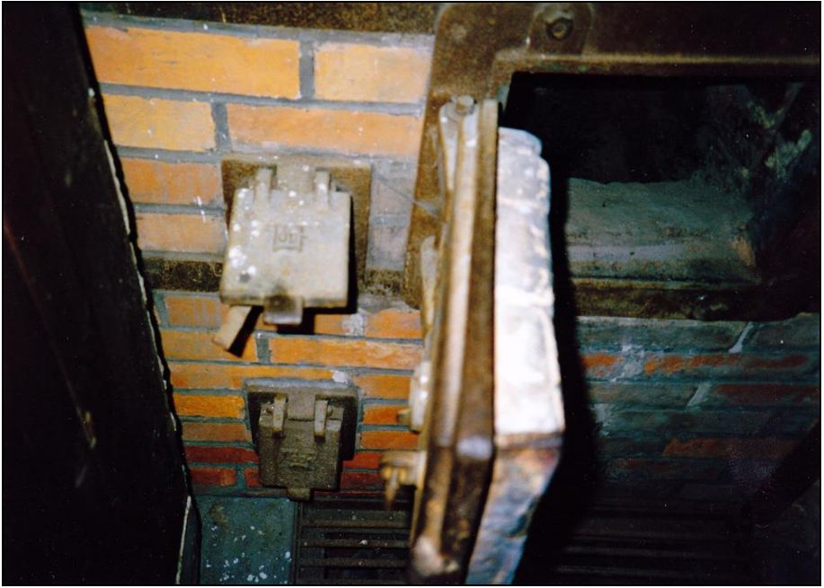
Photograph 39: Left-hand gasifier: large coke-loading door (right), small doors for the primary air to the hearth (bottom) and the primary air to the gasifier (top).
