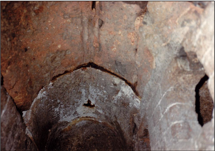
Photograph 19: Left-hand muffle: Vaulted muffle ceiling with the outlet of one of the pipes connected to a blower.
