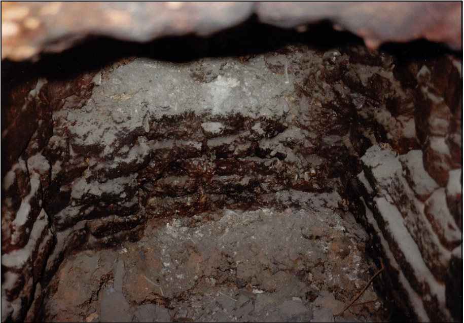
Photograph 164: as above; inside of the gasifier. The masonry shows signs of fusion.
