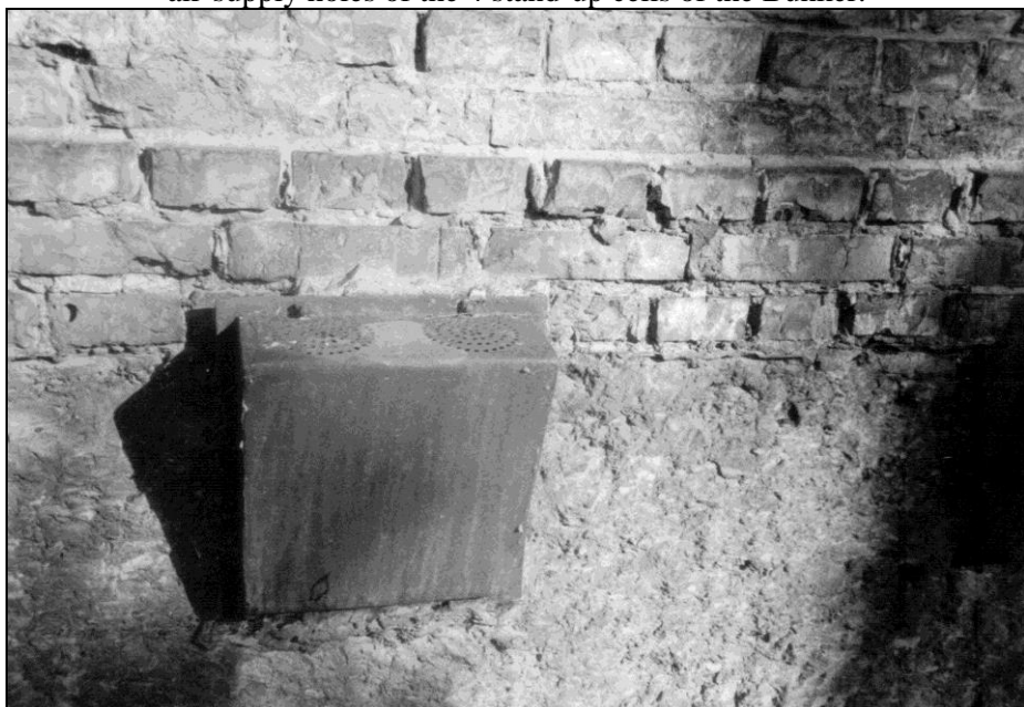
Photo 31: Block 11, outside, wall facing SE, close-up of one of the sheet metal boxes.
