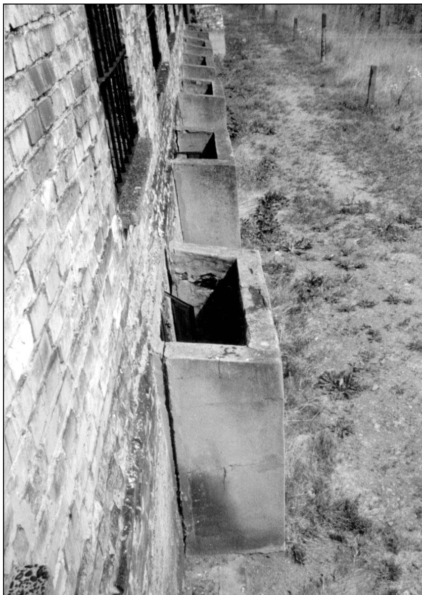
Photo 27: Block 11, wall facing SSW, close-up of concrete covers surrounding the windows of the Bunker cells.
