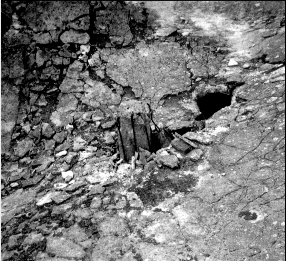
III. 8: Morgue 1 of Crematorium II at Birkenau. Concrete pillar protruding from concrete roof slab and the crack produced by the pillar. August 2000. © Carlo Mattogno.
