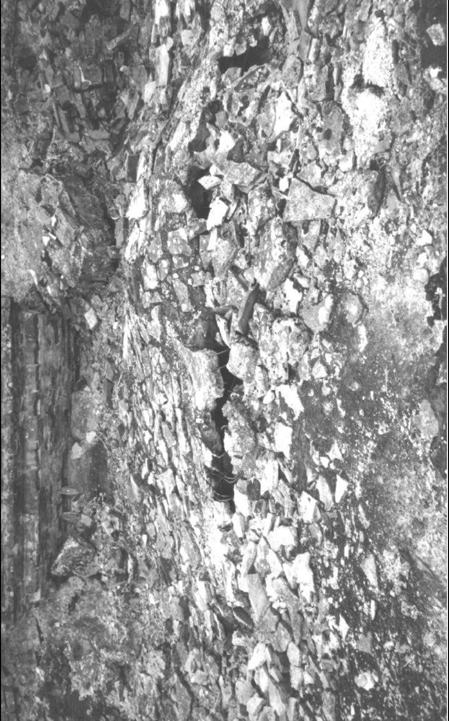
III. 33: Concrete roof of Morgue 1 of Crematorium II in August 2000. Line of the crack, to which Provan's opening no. 8 belongs – to the right of this photo (see photo 34). © Carlo Mattogno
