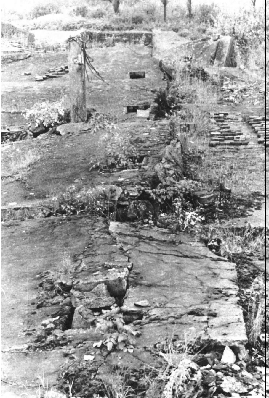
III. 14: All five ventilation openings of the ceiling of the furnace room of Crematorium III. Photo by J.-C. Pressac.
