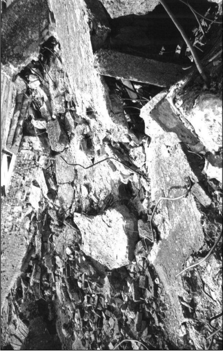
III. 9: Round opening for the pipe of the ventilation through the reinforced concrete roof of Morgue 2 of Crematorium II in Birkenau. August 2000. © Carlo Mattogno.
