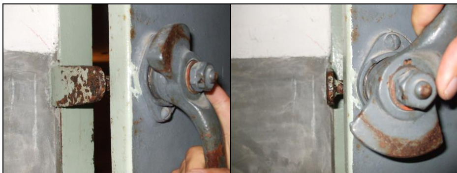
III. 28a & b: The doors to the alleged gas chamber at Dachau cannot be closed nowadays: missing closing mechanisms and blocking steel pins welded to the frame prevent this.
