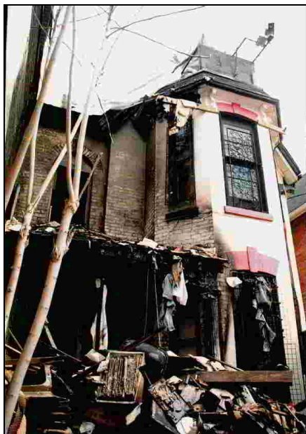
III. 232: Fire damage to the Zündel house after the arson attack on May 7, 1995. © Ernst Zündel
