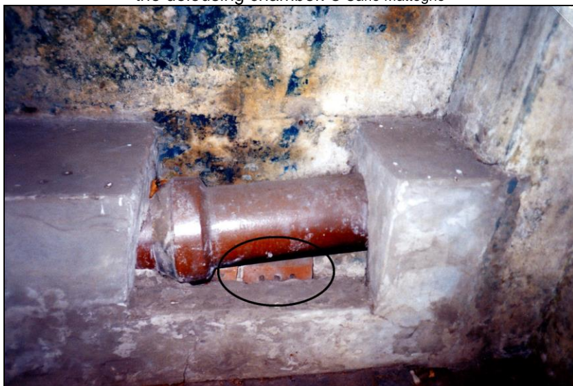
Photo 8: Delousing chamber at Stutthof, interior view, west wall; cast-iron connection pipe to the stove located outside the delousing chamber and used to heat the air inside the chamber. The pipe was originally surrounded by masonry similar to that visible in the photograph, but of perforated brick. One of these bricks is still visible today, underneath and behind the pipe (circle). © Carlo Mattogno
