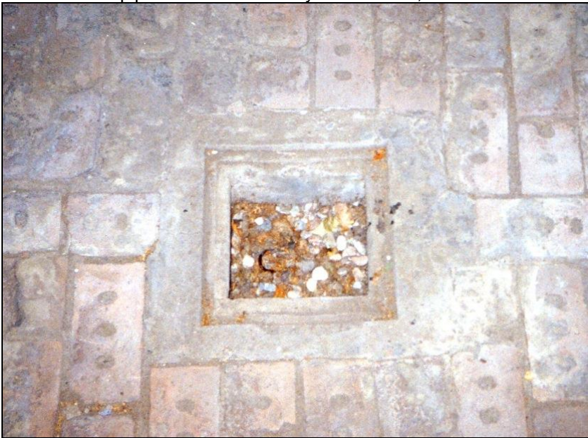
Photo 13: Delousing chamber at Stutthof, interior. Drainage shaft in the middle of the brick floor underneath the Zyklon B introduction hatch. © Carlo Mattogno
